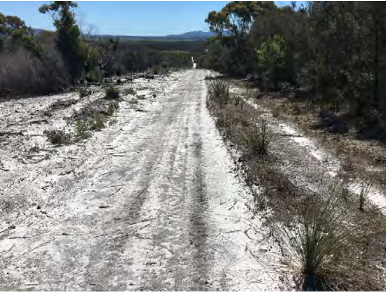
Road access and underground water pipeline from Taswater treatment plant (at Lady Barron Road in the distance) to new holding tank
